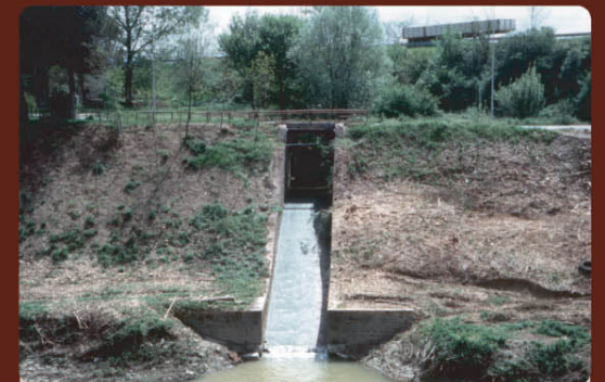
Immissione con scivolo a sagoma parabolica cicloidale del Rio Sellina Hand-built masonry weir-inflow with cycloid parabolic slide at the Rio Sellina
